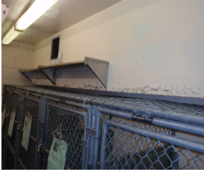
Peeling Paint Above Kennels Located In the Adoption Room at the Staten Island Shelter
