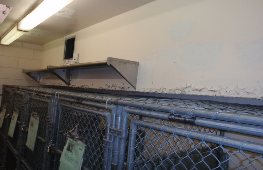
Peeling Paint Above Kennels Located In the Adoption Room at the Staten Island Shelter
